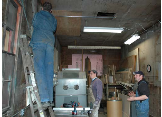
The Roundhouse woodshop gets a long-overdue upgrading by Fraser Ostell (on ladder), Dave Marentette & Skylar Reyburn.
